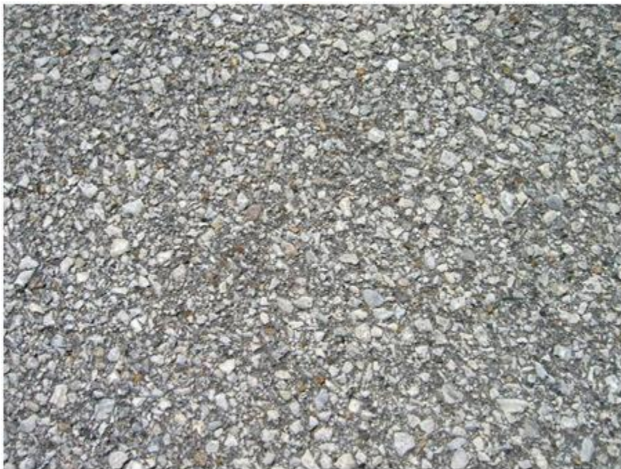
Fully Weathered Old Surfacing On the Verge to Break
