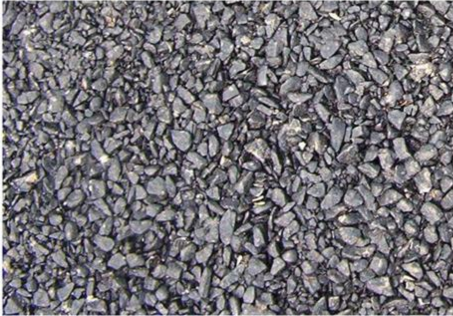
Less Dense Bitumenous Mix, Vulnerable to weathering due to accumulation Accumulation of Water, Free Access to Sun Light and Air .
